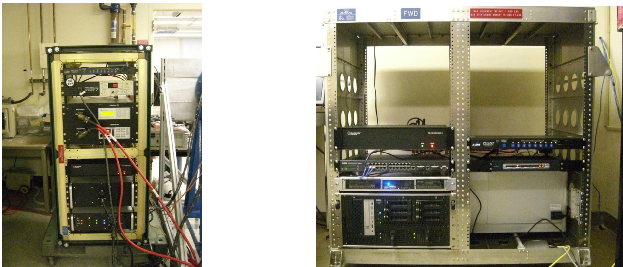
Figure 10: CW rack (left) and PI rack (right). The former contains instrument electronics and PI rack holds computers.
